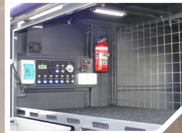
Power Switch Board
