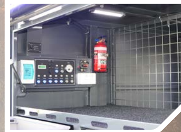
Power Switch Board
