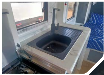
Internal Kitchen Sink
